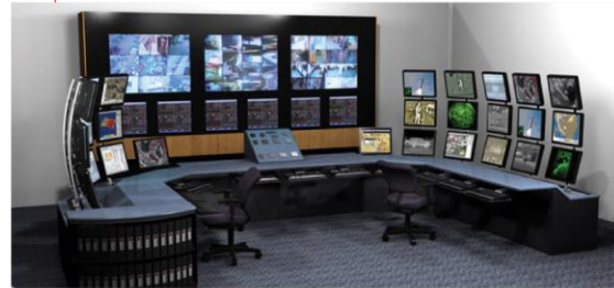
Integration to Standard security Panels (small projects)
